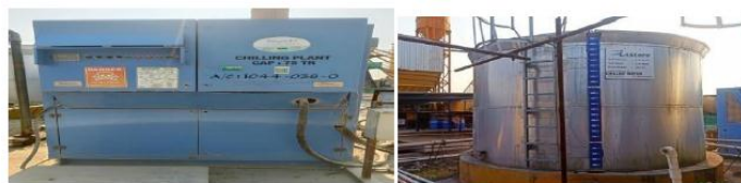
Fig 27: Chilling plant is in working condition-Chilled water stored in Insulated
