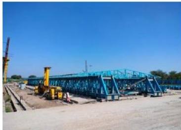
Fig11: Strong back truss attached to Straddle carrier used for lifting moulds & Rebar cage from Jig
