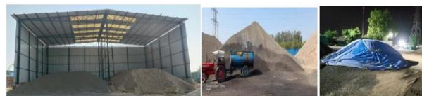
Fig 27: Aggregate kept in shed -Water sprinkling on aggregate by water tanker-Aggregate covered by tarpaulin sheet
