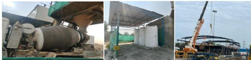
Fig 30: Transit Mixer's drum wrapped with wethessian cloth Admixture kept in shed. Shed provision during
