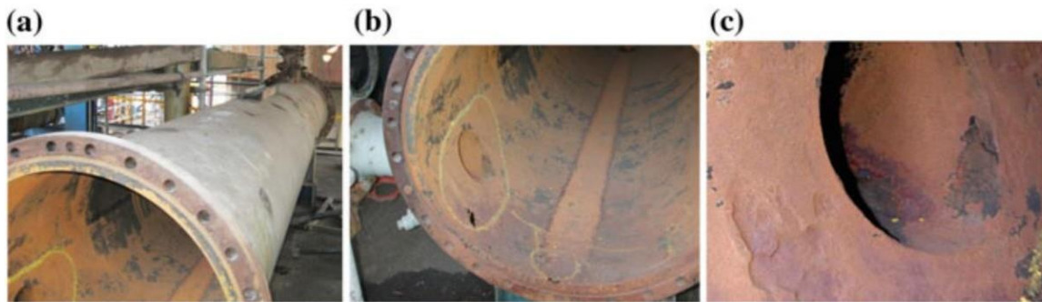
Figure 3(a) shows the second vacuum condenser's shell's damaged inner surface. Localized corrosion from the second vacuum condenser can be seen in (b,c) close to the water condenser.
