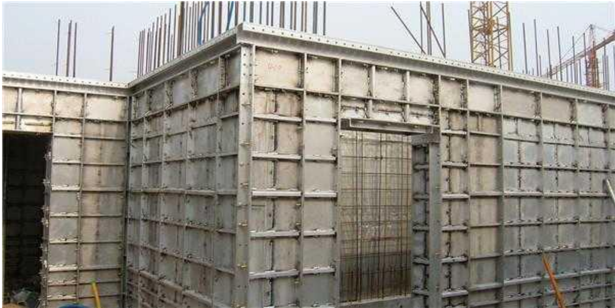
Fig. 2. vertical formwork systems used to form the vertical supporting elements of the structure, e.g., columns, core walls, and shear walls.
