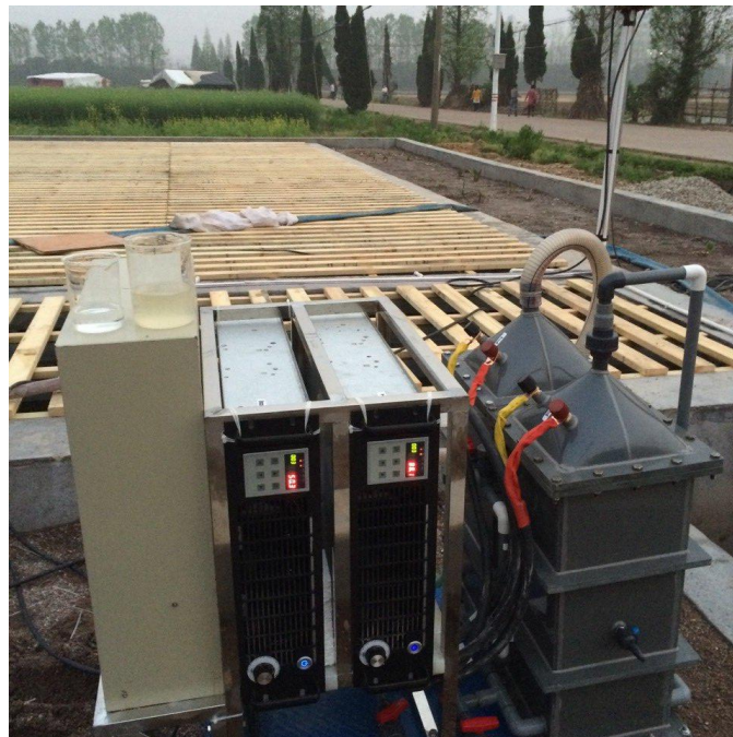
Fig. 4 Wastewater treatment unit by electrocoagulation and electrooxidation
