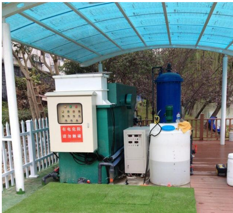
Fig.6 Wastewater treatment device in Hangzhou City for a food market
