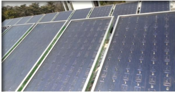
Fig. 2 Experimental Demonstration of an Evacuated FPC at Solar Energy Centre
