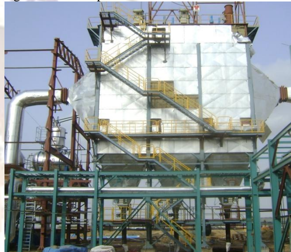
Fig.10 Onsite Equipment of ESP
