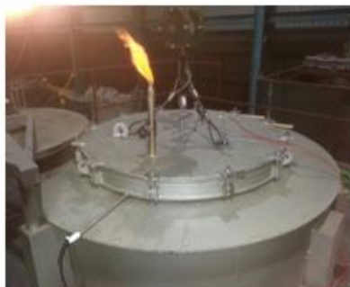
Fig. 1.2 – Excess Hydrogen burnt through Furnace lid.
