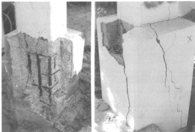
Figure 10: damaged concrete column showing large spalls and cracking
