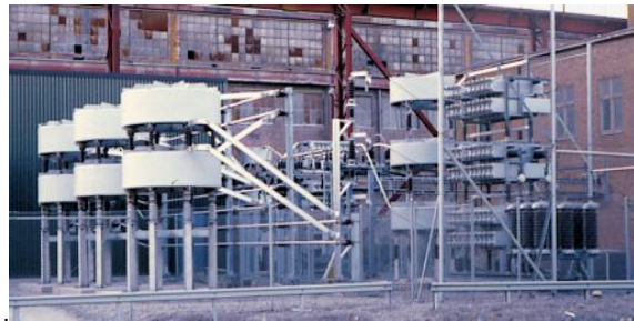
STATIC VAR COMPENSATOR CONNECTED TO BUS TERMINALS
