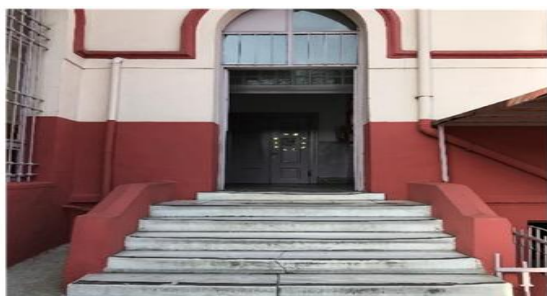
Figure 5. Deteriorations At The Şemsipaşa Primary School
